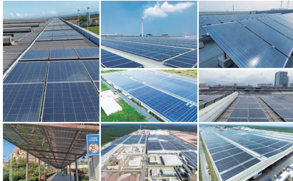
SOLAR PANELS IN INDUSTRIAL PARK
